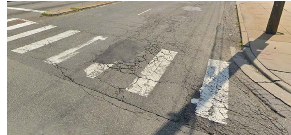
Potholes on Rte 1 at Bells
