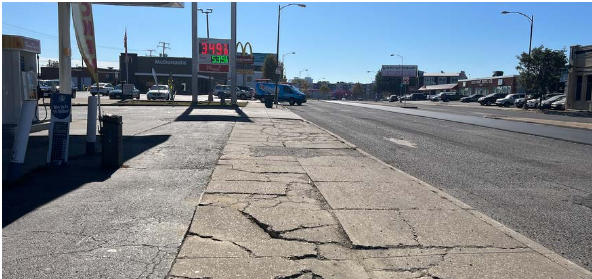
Cracked sidewalk on Chamberlayne
