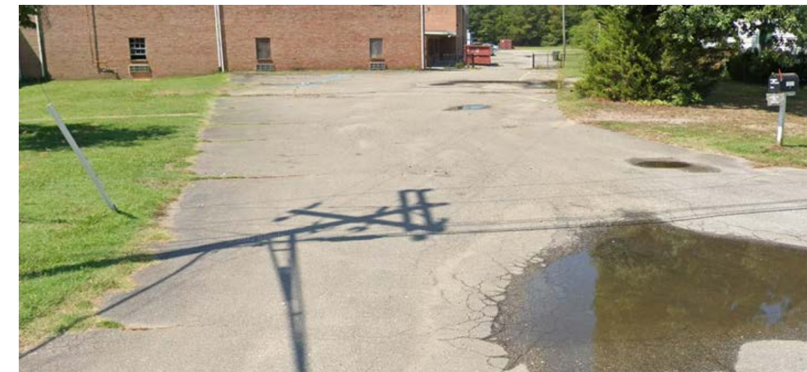
Potholes near Southside Community Center
