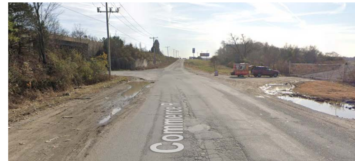
Pavement condition on Commerce Rd
